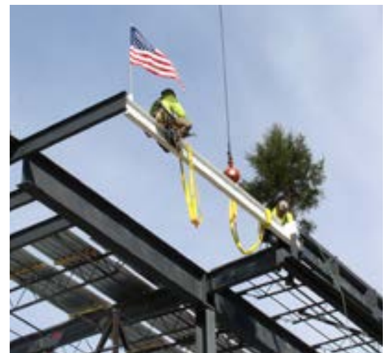
Construction crew workers secured the beam into place atop the three-story framework.
